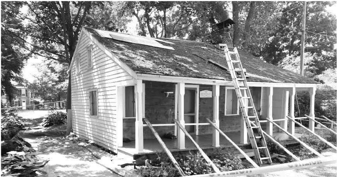
Our Thomas House roof is being prepared to receive a fresh new treatment. photo Mark Verlinden
