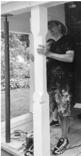
Mark Verlinden, at left, makes sure the new post at the Thomas House is vertical.
